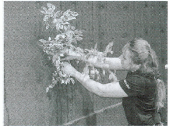
Monique Lee of Nedlaw Living Walls installs plants Wednesday on the newly redone living wall at Guelph City Hall.
